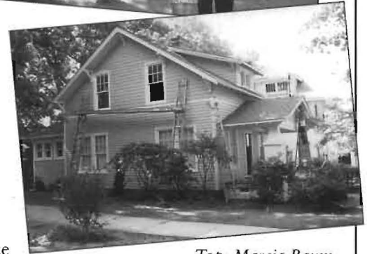
Top: Marcia Baum and Sean Frelke in front of their rehabilitated Elm Street house. Bottom: Charlie Wanta completes exterior work at 601 Cutler.
